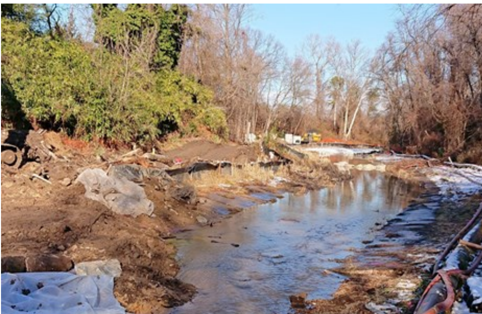
Multiple sediment controls in place, including access road with silt fence, a 12" pump around and, in the foreground and background, white plastic to prevent shearing of the newly graded channel.
