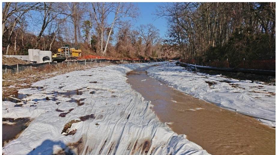
Impermeable white plastic protects the newly graded channel from eroding while work continues upstream.
