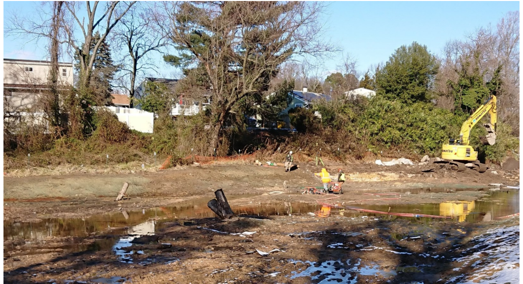
A portion of the stream channel being actively graded. Water is being pumped around the work area to allow machinery into the channel. Workers can be seen carrying one such pump.
