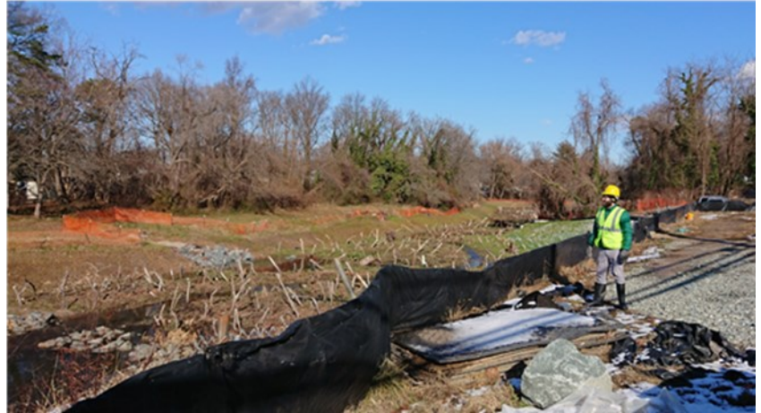
PGSCD Engineer, Spencer Evans observes a restored wetland floodplain intended to mimic natural features that reduce flow velocities and provide habitat for fish and insects.
